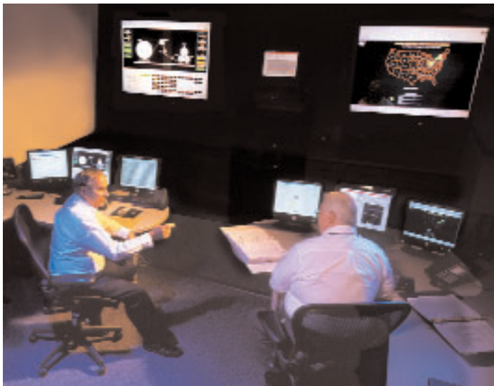
High speed plant floor networks and telecommunications technologies make it possible for process and controls specialists at Rockwell Automation's In.Site Command Center in Cleveland, Ohio to remotely monitor real time production data from plants located almost anywhere in the world, 24x7x365.
