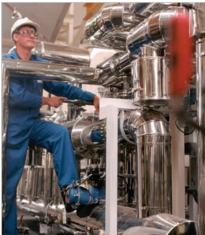
The life of most equipment requires periodic maintenance. At ChiRex Ltd's multi-product facility in Annan, Scotland, a process operator monitors solvent distribution pipework.
