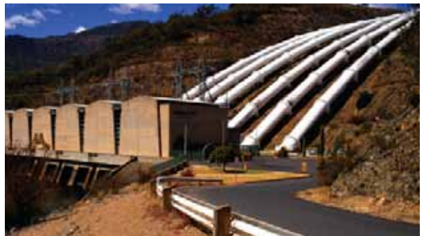
Snowy Hydro's seven-year, A$250 million 'Scheme Modernisation Project' upgrade is the scheme's first major overhaul
