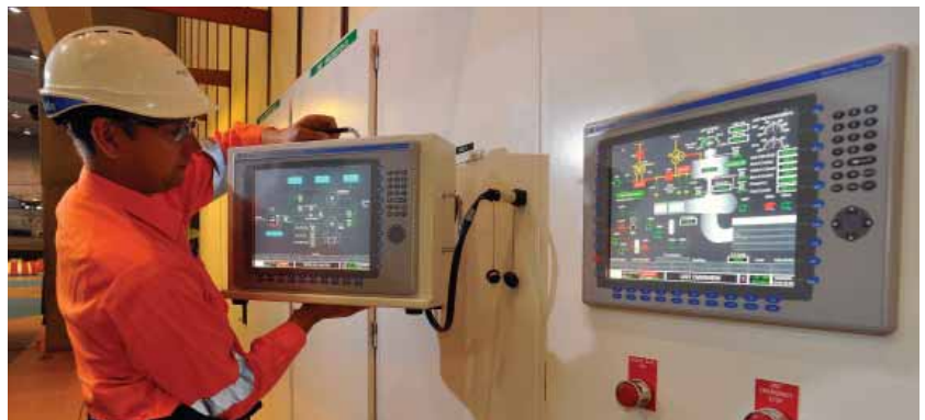
The controls upgrade included the replacement of legacy relay logic controls and analogue gauging, with state-of-the-art PAC and electronic operator interface technologies.
